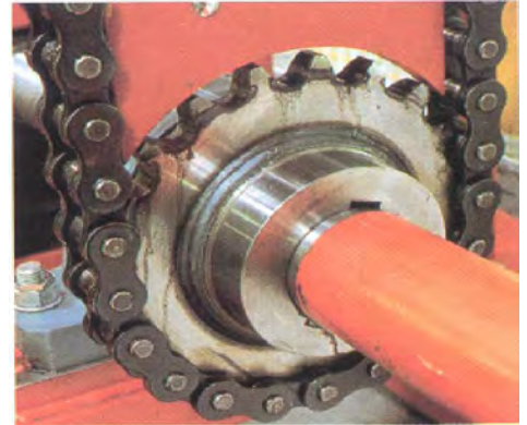
Deflection Chain Wheels in Car Manufacturer Paint Shop
